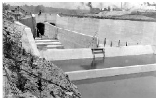
removed just before water was allowed to enter. The finished permanently open outlet conduit at Englewood Dam is shown on June 28, 1919 (right), just before water was allowed to enter. View is looking upstream from the end wall at the base of the spillway toward the dam, showing the stair-step structures on the spillway's floor (water would flow toward the viewer and off to the lower right).
